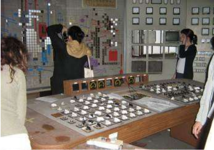
Figure 3: The Central Controls Room
